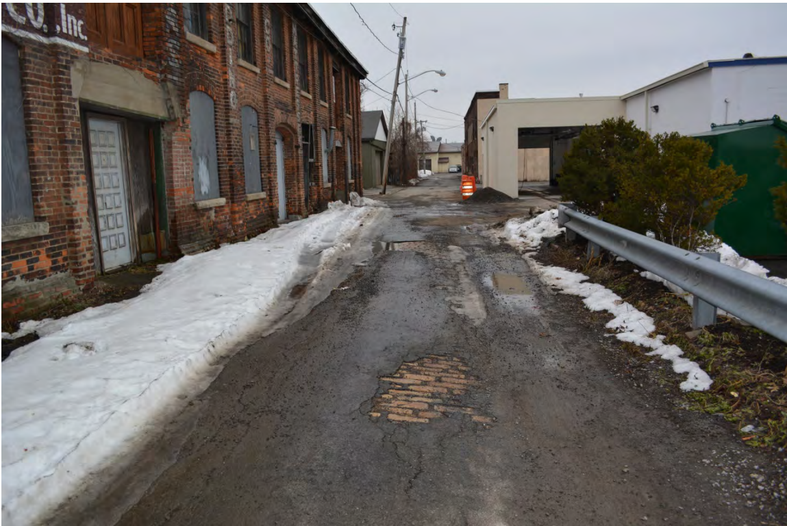
Photograph 16. View from east end of Carton Avenue, facing west. Note, exposed sandstone pavers in foreground (Panamerican 2018).
