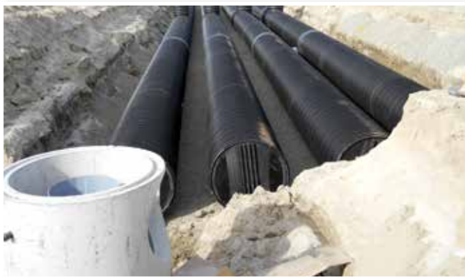
CDS pretreats a rainwater harvesting cistern.
